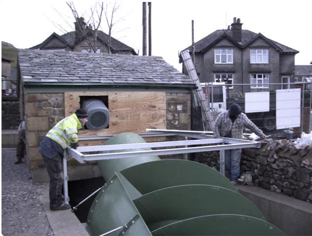
The Archimedes Screw in the Settle Hydro run-of-river scheme
